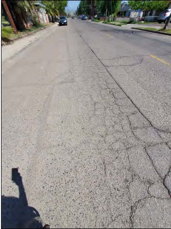
Figure 3: Subsidence of UUI on Harvard Ave
