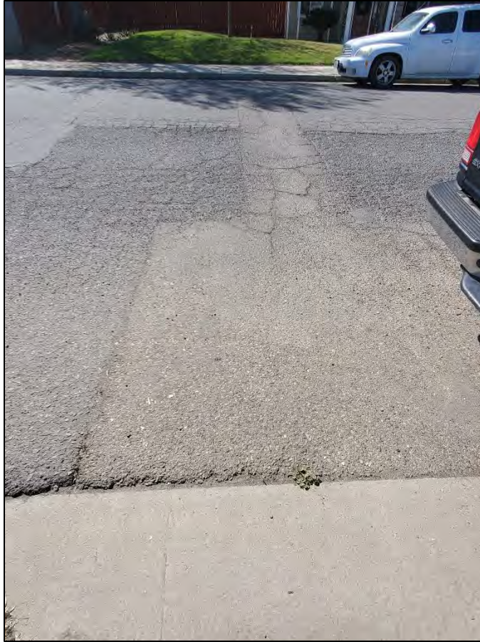
Figure 2: Trench Patch on Hickory Street
