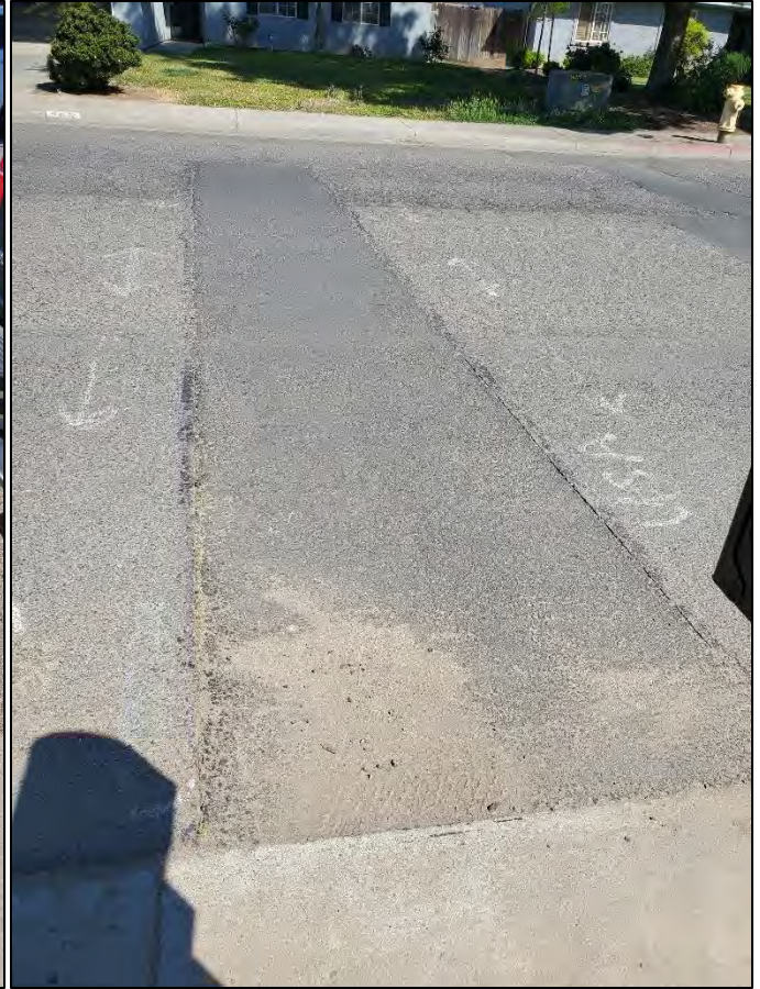
Figure 1: Trench Patch on Hickory Street
