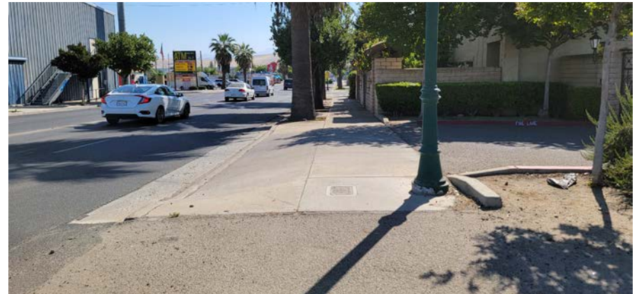
Sidewalk maintenance needed in various sections
