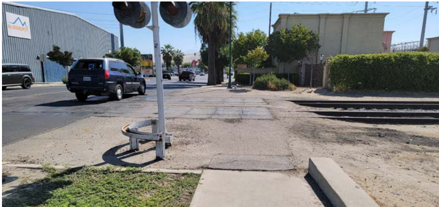
Sidewalk maintenance needed over at-grade railroad crossing
