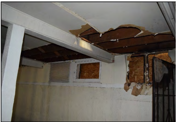
Basement Fire Damage
