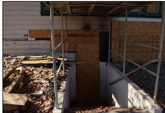
Front View – Fire Damage
