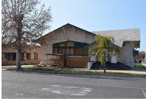
Front View – Exterior Fire Damage
