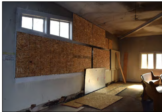
Sanctuary Fire Damage
