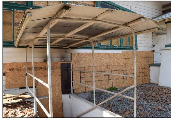
Front View – Fire Damage
