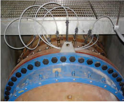
Westfall Model 2800 Static Mixer in-line at Sebago Lake Water Treatment Facility.
